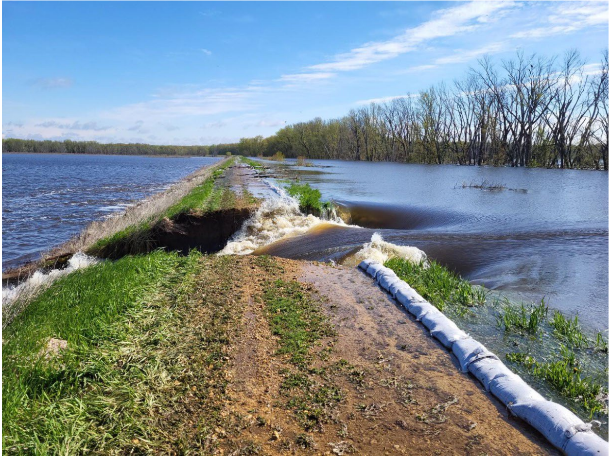
Figure A-11. 2023 Green Island Levee Breach near Brown's Lake around Sta. 400+00.
